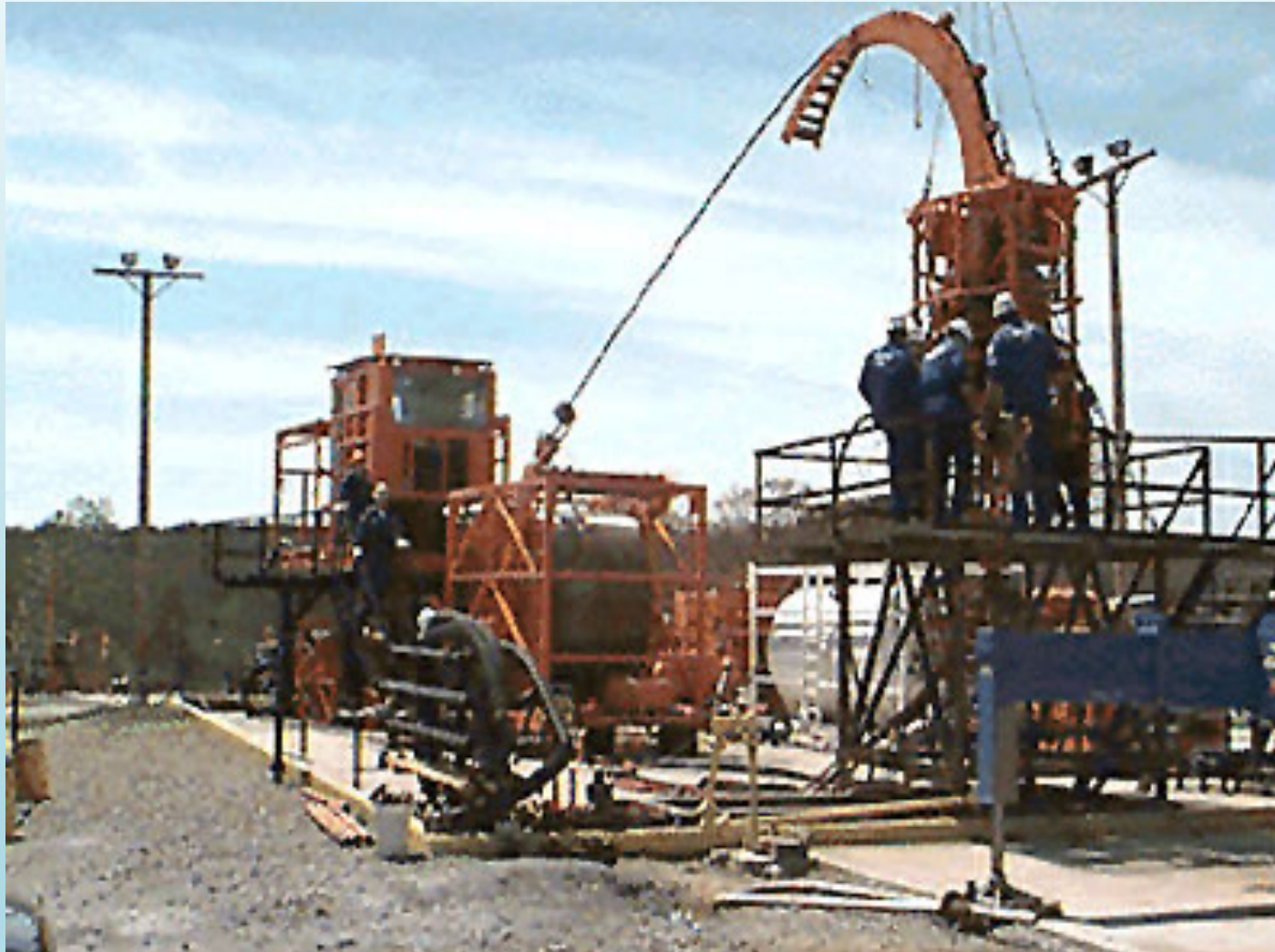
Figure 8 CT surface operation unit - string and associated equipment
